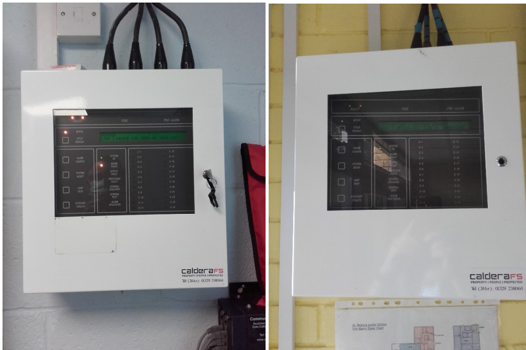
Figs 6&7 – Main Panel and Repeater Panel respectively
